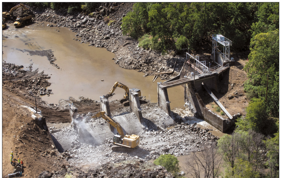
Workers demolish Copco No. 2, the first of four Klamath River dams to be removed. Shane Anderson/Swiftwater Films photo
